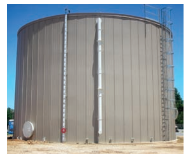
Fire Protection Tank
